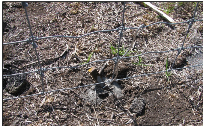
Proper use of concrete pin to anchor fence down. Notice the pin does not contact the woven wire.
